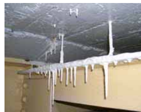
床版下面の遊離石灰
